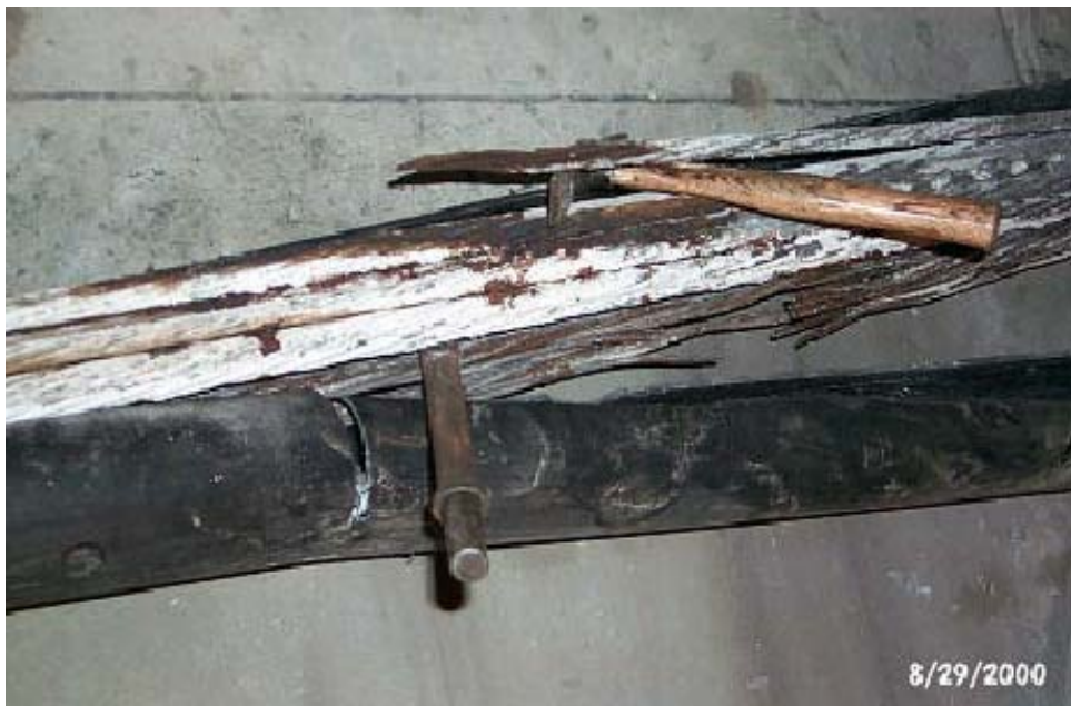
Figure 1.9: Failure of Tendon 28-6 on the Mid-Bay Bridge (FLDOT 2002)
