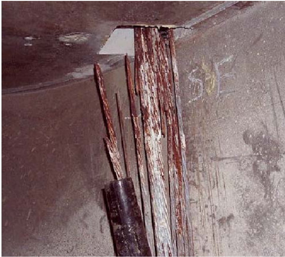
Figure 1.12: Tendon Corrosion inside the Sunshine Skyway Bridge Piers (FLDOT 2002)
