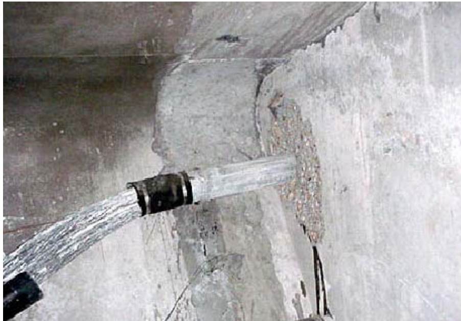
Figure 1.10: Failure of Tendon 57-1 on the Mid-Bay Bridge at Expansion Joint Diaphragm (FLDOT 2002)
